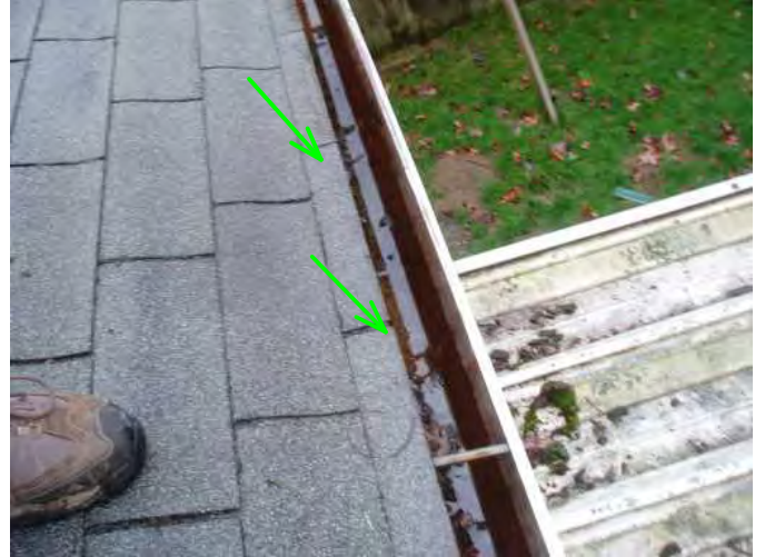
gutters are noted draining well as it is a rainy day today...clean as well...
