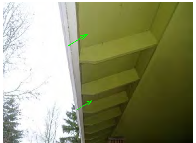
soffits under overhang of roof are noted solid and sound...no soft or rotted wood noted...good..
