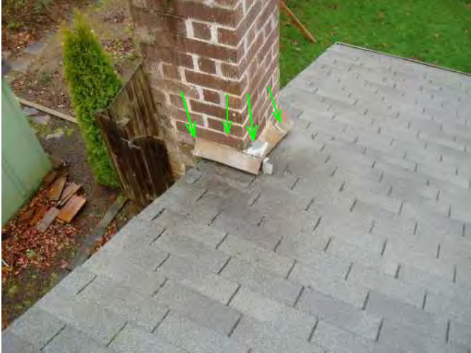
brick chimney is flashed with step flashing and covered well with counter flashing...no apparent leaking noted...
