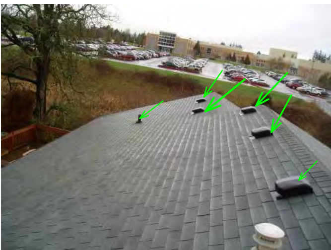
back of home facing west shows vents for attic are secured and plumbing vents are flashed well and sleeves are fine...
