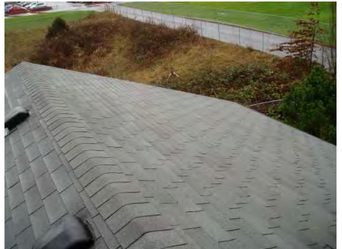
all shingles are clean and performing drainage well...front northwest area of home...
