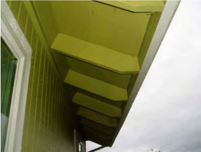
same noted here at soffits at back of home...good...
